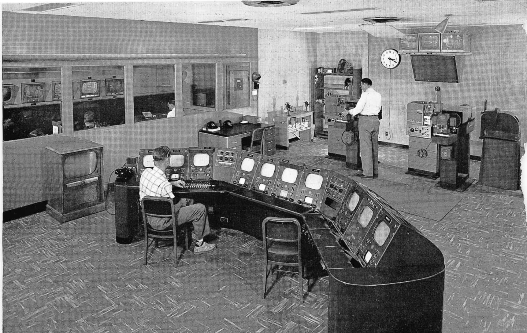
FIG. 9. WHIO's TV Master Control Room contains not only master switching equipment but also all camera controls and film projection equipment. Studio 2 camera control units are at left of main console; Studio 1 camera controls are at right; film camera controls, preview and line monitors are in the center.
