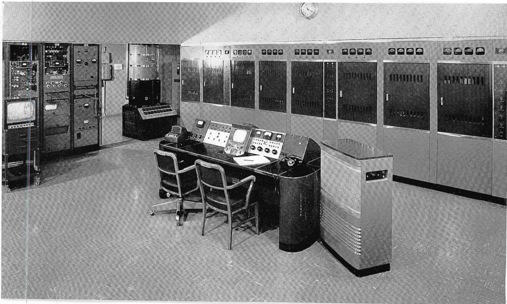
FIG. 12. WHIO's RCA TT-25BH Transmitter is the center of a U-shaped equipment layout. Left of the U consists of racks for input and test equipment. Right of the U will be formed by WHIO's original RCA TT-5A Transmitter which will be moved from studio building and used as an emergency unit.
