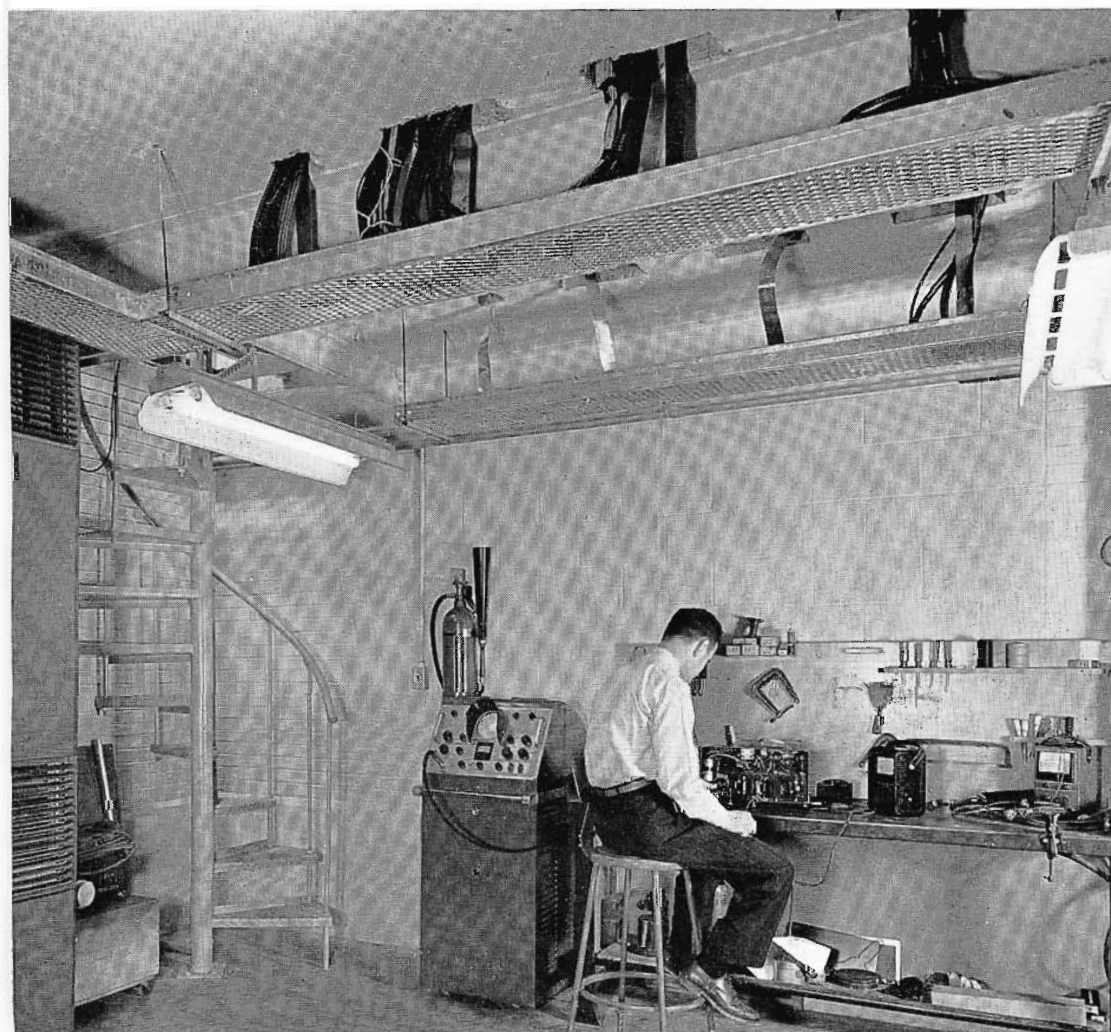
FIG. 10 (below). View of the engineers' shop and equipment room. Note cables coming through floor from master control directly above. These are carried in cable baskets to drop-out locations above equipment racks which are out of sight at left.
