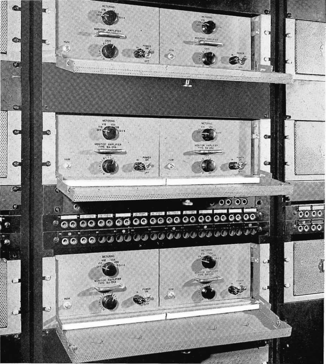
FIG. 6. View showing BA-24A Monitoring Amplifiers at NBC Studios in New York.
